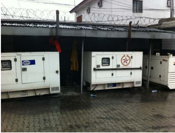
40 & 60 KVA GENERATING SETS
